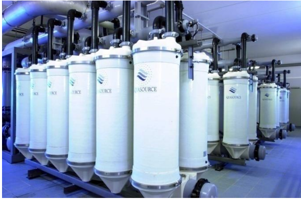
Drinking water station (24,000 m 3 /day) in ROUEN with 4*24 modules of 125 m 2 surface area. Commissioned in 2000
