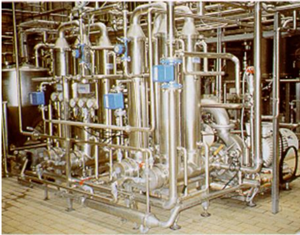
Microfiltration unit for whey treatment
